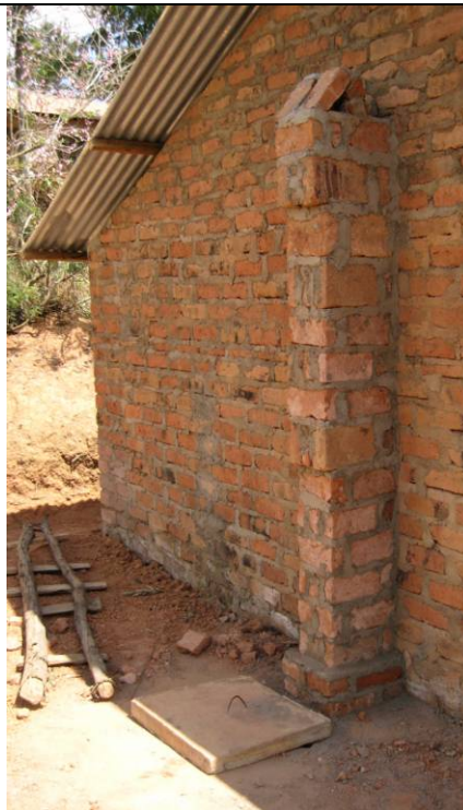
Tank cover and air outlet at the backside
